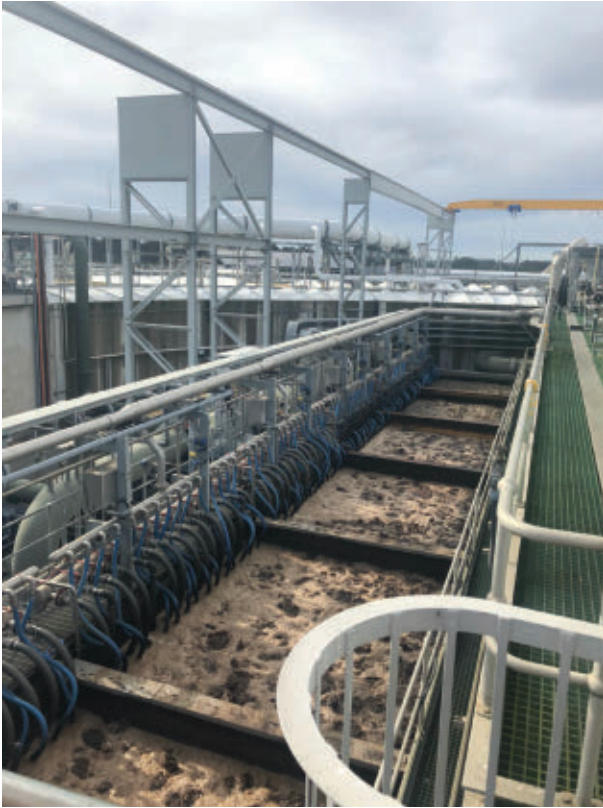
Figure 1. Membranes submerged in the activated sludge of an MBR
